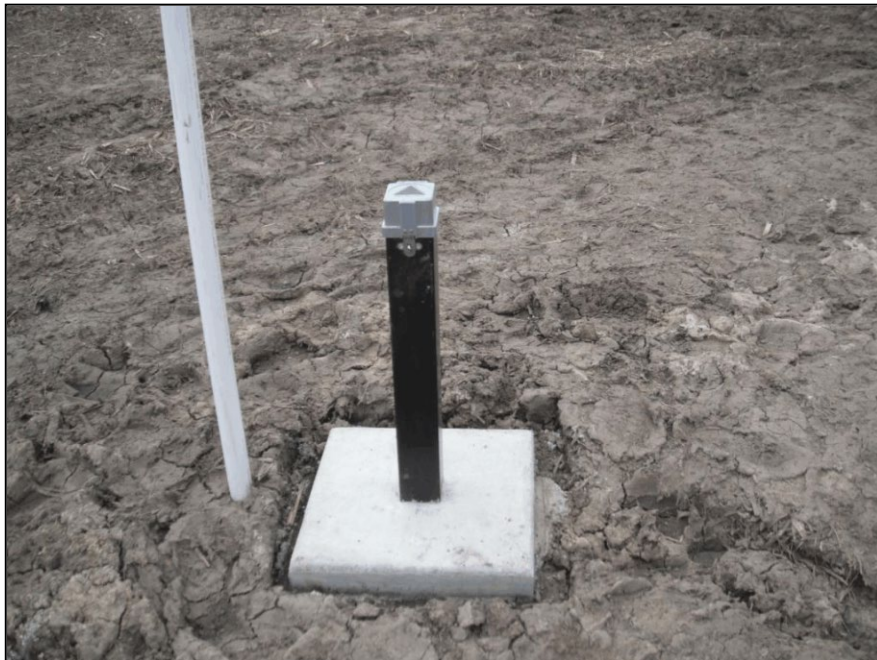
Photograph 2.8-1 Typical Monitoring Well
