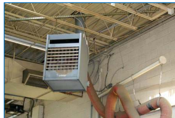
Infrared Heater - Lorton, VA
