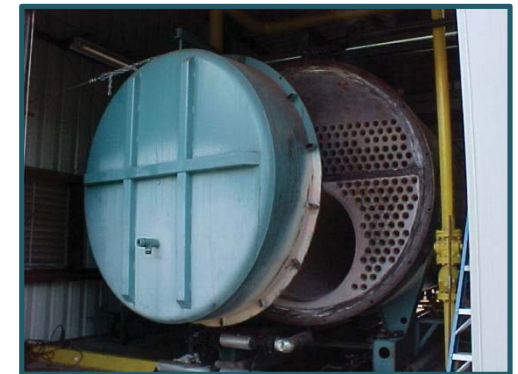
Boiler – Raleigh, NC
