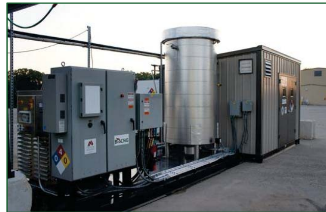
BioCNG System Dane County, WI
