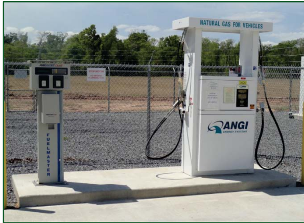
CNG Fueling Station St. Landry Parish, LA
