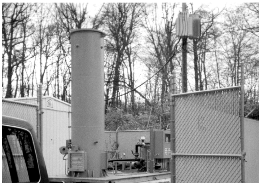
Figure 5-8. Small Skid-Mounted Enclosed Ground Flare.
